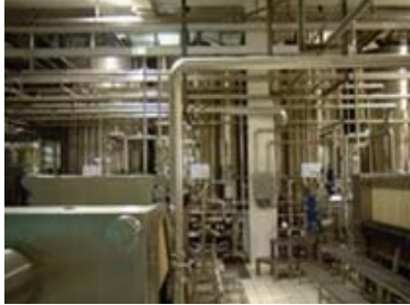
Fermentation piping system
